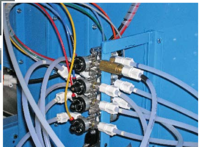
Automatic stain color change manifold with circulating stain lines — Color Change Manifold
