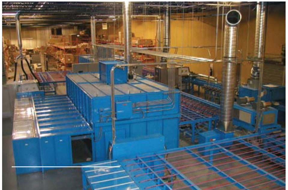
ABC Millwork's new finishing system's footprint is smaller than before and allows it to cut down its throughput times and eliminate the need for racking pieces between steps.
