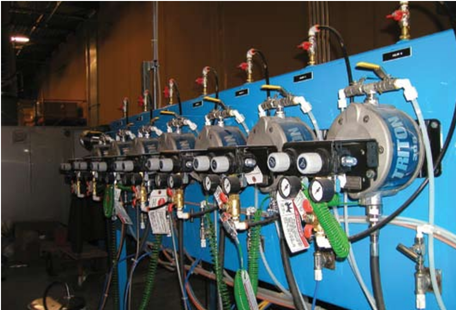
ABC Milwork uses individual stain pumps that feed the color changer. With its new system, colors can be switched in as few as 30 seconds.
